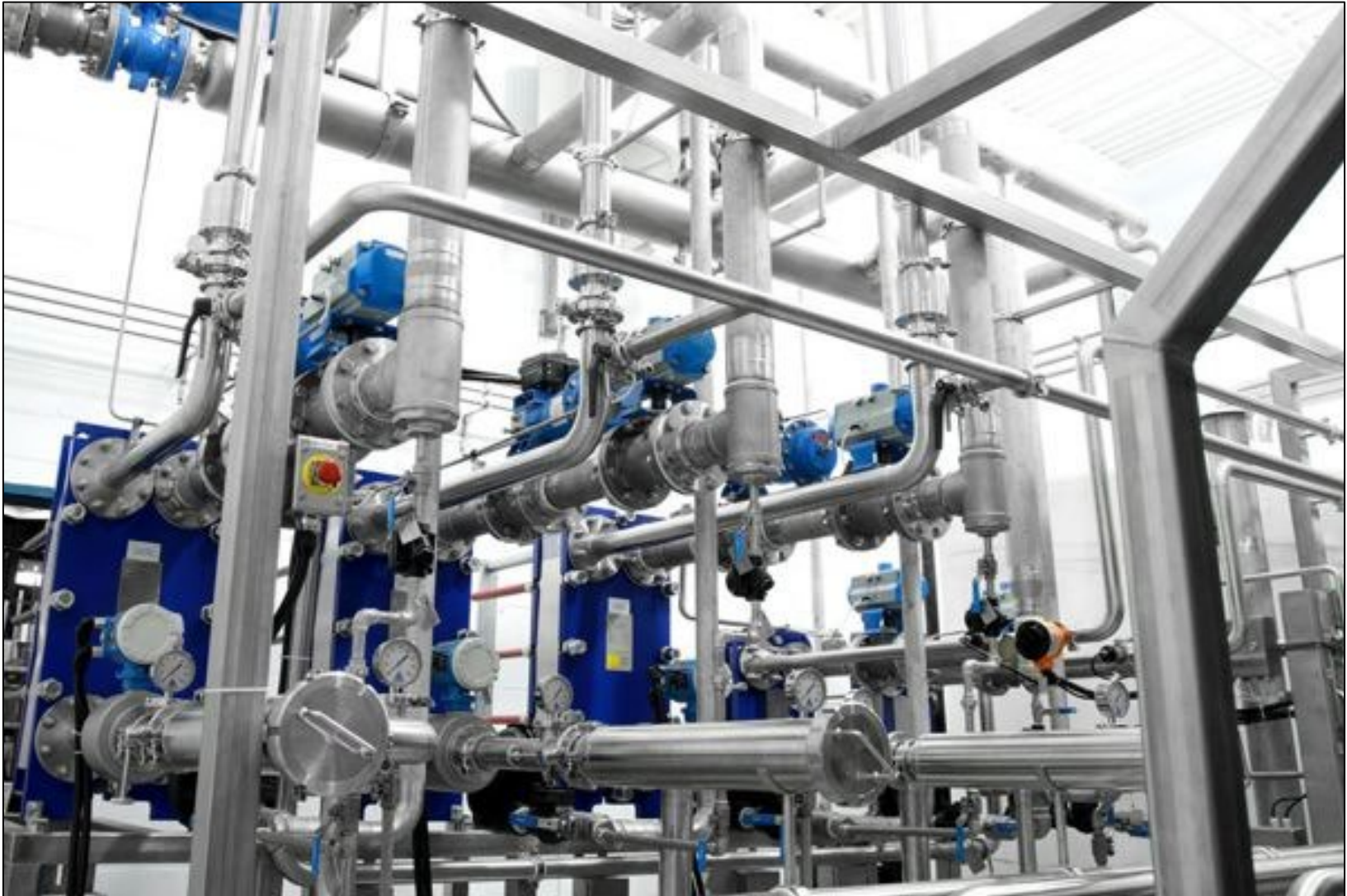
Stainless piping system
